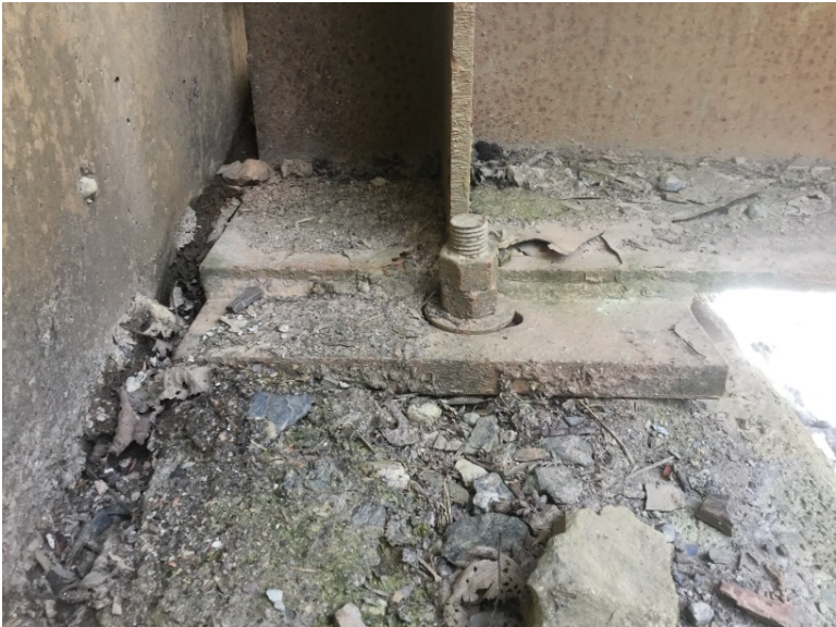
Slotted bearing holes at right bank
